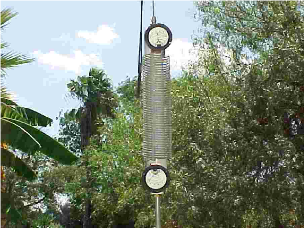
Figure 48. RF ammeters reading 100 MA on the bottom and 42 MA on the top of the loading coil.
