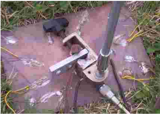
Figure 26. Base mount over the radial system.
